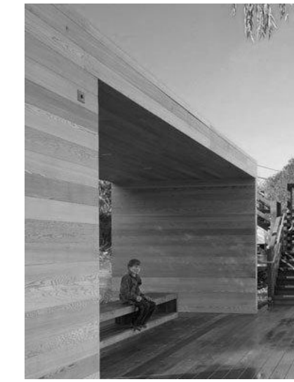
SIDING 1"x4" V-JOINT T&G HORIZONTAL CEDAR SIDING, WHITE WASH, CLEAR SEALED (CONTINUE INTO INTERIOR)
